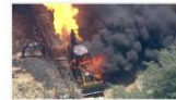
A fire erupts in Woodland Hills after a backhoe struck a gas line and ignited it on Wednesday, Aug. 3, 2016.
